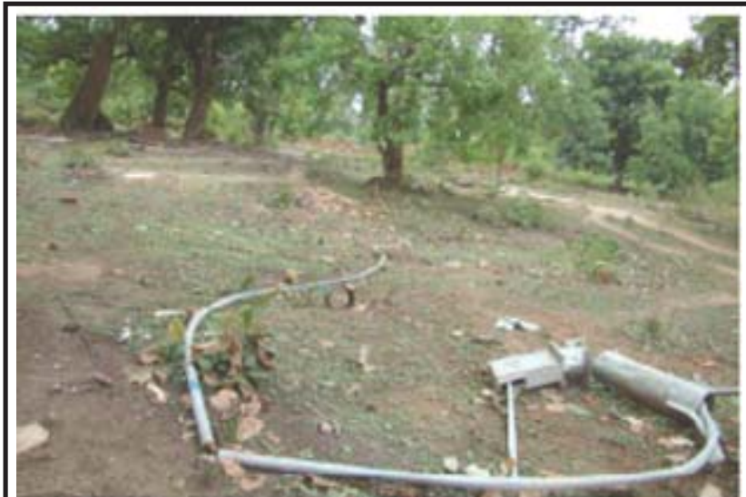
During the demolition, the Administration did not even spare the hand pump, though it was installed by the Government itself.
