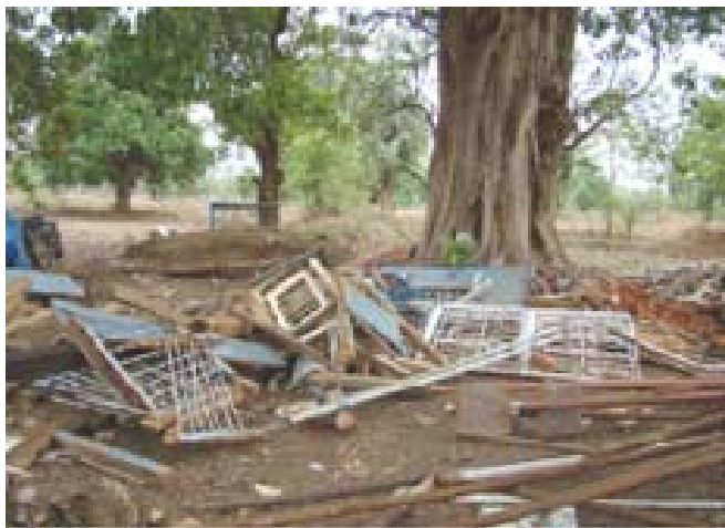
A beautiful site with numerous trees and structures made with local artistry destroyed during demolition.
